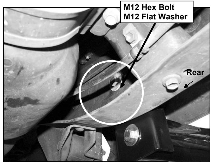
(Fig 6) Back view of driver side-rear frame channel pictured(example only)
