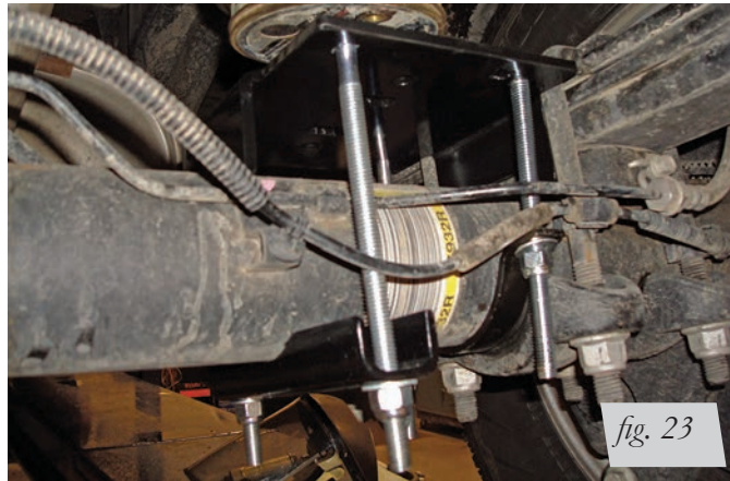
Right side (passenger) view towards rear of finished installation torqued to 10ftlbs.
