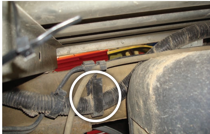
Inside frame, left hand (driver side) view
