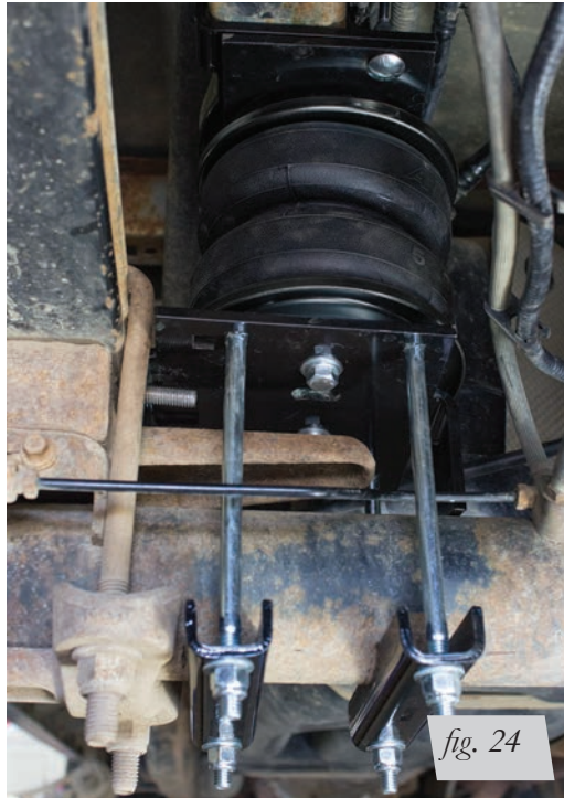
Left side (driver): rear view of installation.
