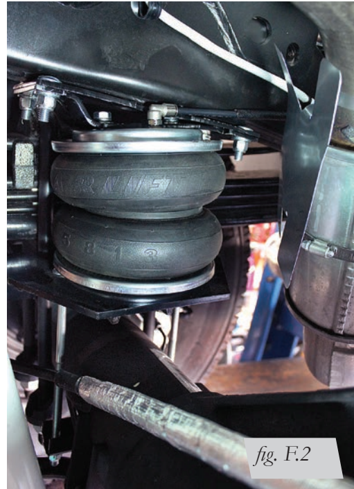
Passenger's (right) side inside frame view of kit installed.
