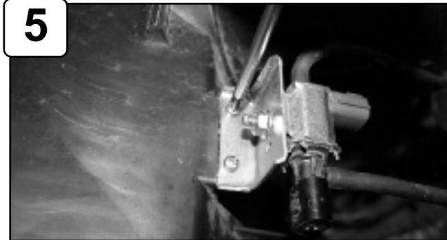
Loosen VSV sensor using phillips screwdriver on back of air box. Carefully remove. Remove air box out of vehicle.
