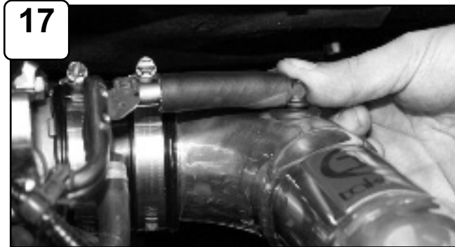
17 Using the supplied 3/8" elbow, hose and grommet, reattach the crank case line. Re-connect MAF sensor harness and battery terminals.
