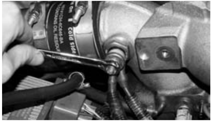
5- Using a 10mm wrench, remove the heating element wires.
