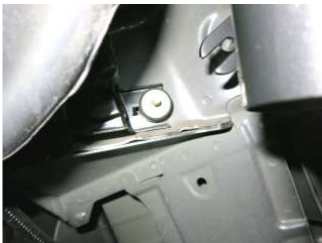
a. Install the provided rubber bushing into the bolt location that was removed in step 2l.
