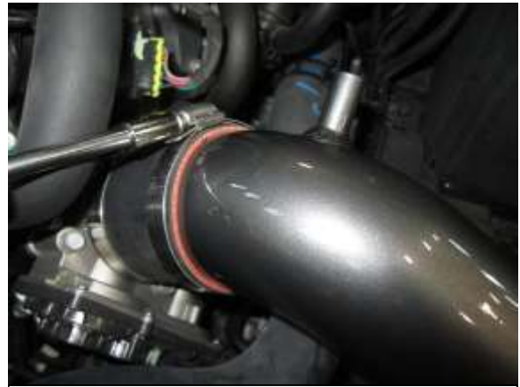
F. Once properly seated, tighten the second hose clamp at the intake tube outlet connected to the throttle body.
