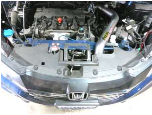
m. Reinstall the plastic radiator shroud you removed in step 2a/b, adjust intake tube for best fitment, then tighten the hose clamp at throttle body coupler and the bolt at intake tube bracket.
