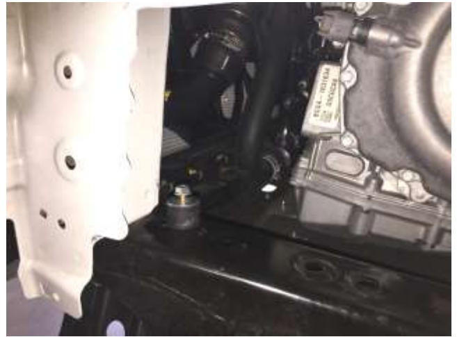
a. Install the provided rubber mount, nut and washer where the resonator support bracket was removed.
